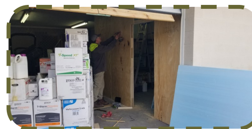
The chemical storage room in the process of being built, pictured above.
